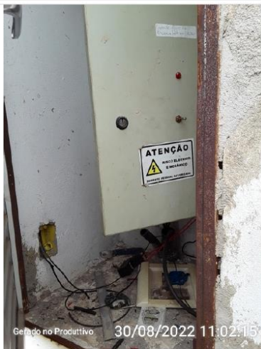
Painel de controle
