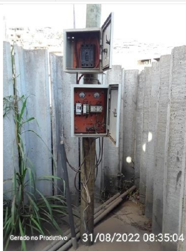
Painel de controle
