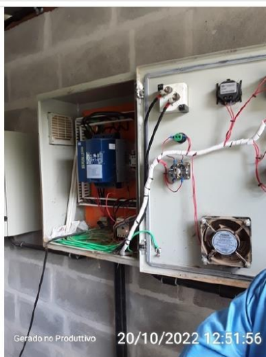
Painel de controle
