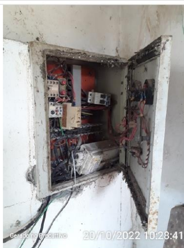
Painel de controle
