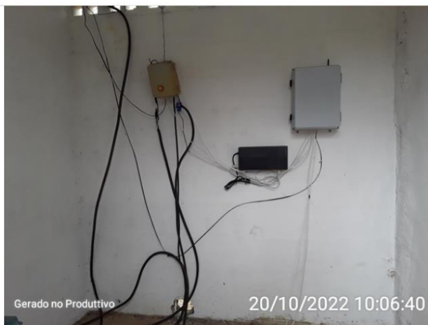
Painel de controle
