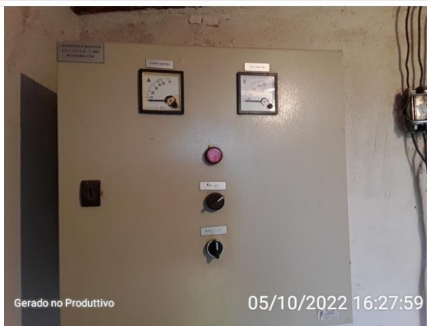
Painel de controle
