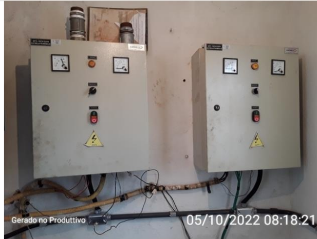
Painel de controle
