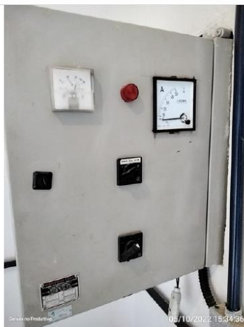
Painel de controle
