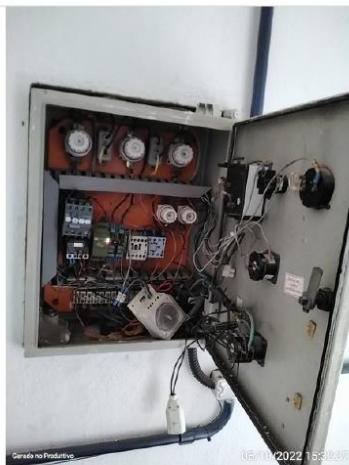
Painel de controle
