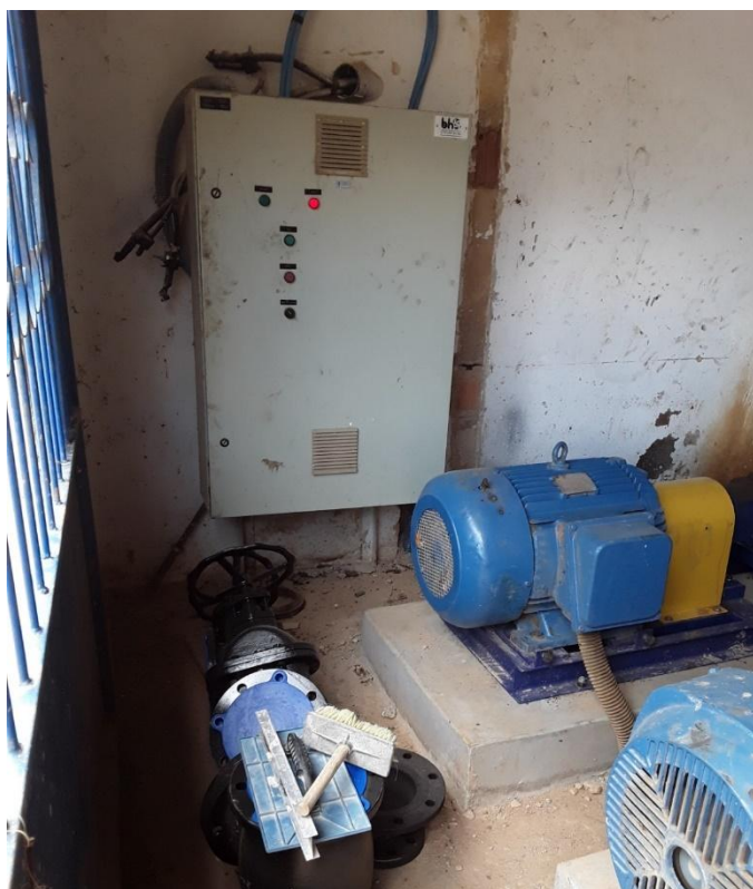
Figura – Painel de controle – EEAB Usina
