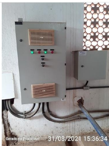
Painel de controle
