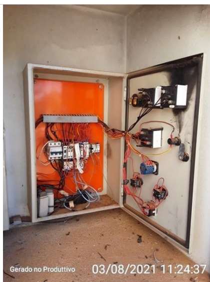
Painel de controle
