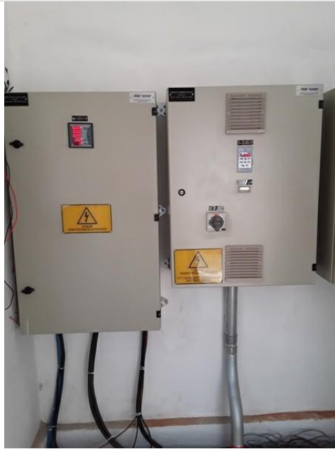
Painel de controle
