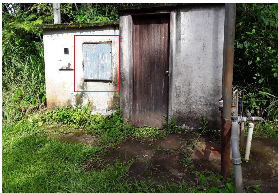
Figura 51 – Painel de Controle – Vila Alves
