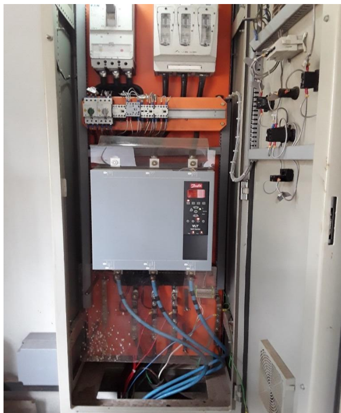
Figura 138 – Painel de controle – Bomba 1
