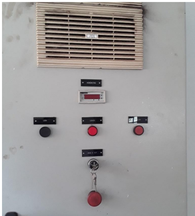
Figura 139 – Painel de controle – Bomba 2
