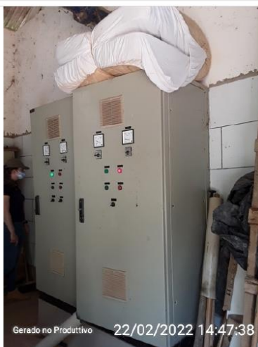
Painel de controle
